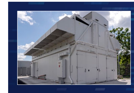
TX-GAIA is housed inside of a new EcoPOD deployable data center, manufactured by Hewlett Packard Enterprises, at the site of the Lincoln Laboratory Supercomputing Center in Holyoke, Massachusetts.
